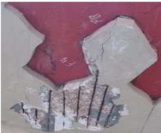
(a) Corroded and spalled weather shade indicating the failure of earlier repair.
