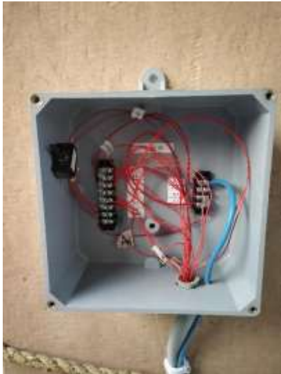
(a) Photograph of the monitoring box
