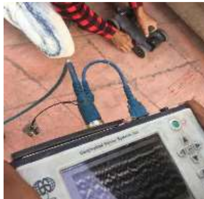
(b) Rebars were located using a rebar locator, and the locations were marked on the sunshade
