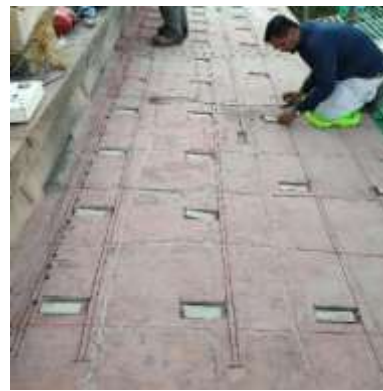
(h) Anodes were placed in the low resistive mortar inside the pockets
