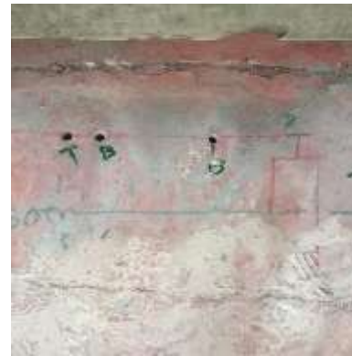
(c) Several 10 mm Ø holes were drilled to establish an electrical connection with the rebars
