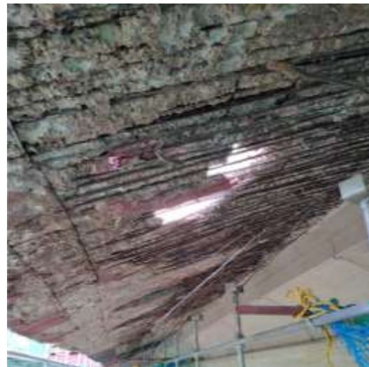
(b) After removing the cover concrete, all rebars were corroded — a classic example of hidden corrosion in a patch repaired area of concrete.
