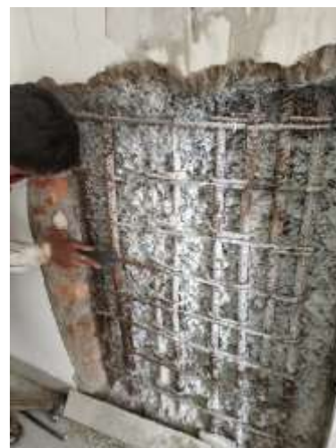
(b) Rebars were corroded when the cover concrete of a cracked RC column –on the 6 th floor of Tower E – is chipped off.
