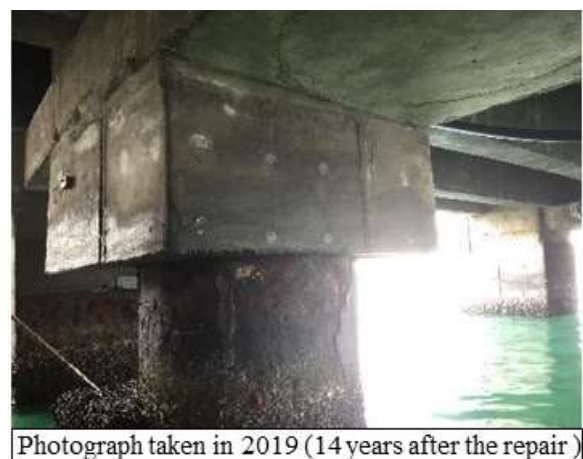
(b) CP protected pier after 14 years
