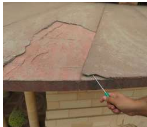
(b) Past repair interventions with polymer-modified cementitious mortar was not successful
