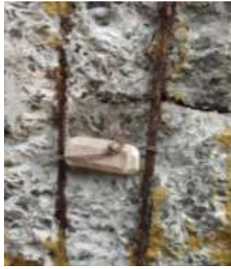
(b) Loosely tied galvanic anodes around the steel reinforcement
