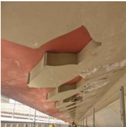
(a) Before removing the cover concrete, the sunshade looked neat and clean from the outside
