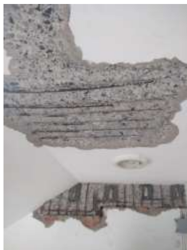
(a) Spalled concrete from a ceiling slab on the 3 rd floor of Tower D
